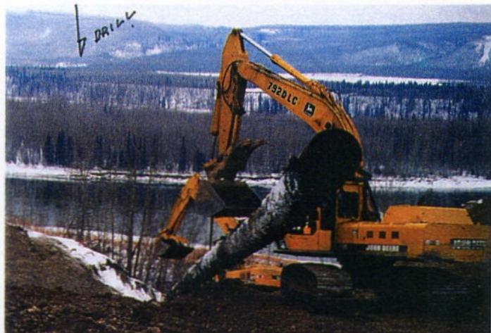
Casing installed on the exit side aided in the recovery of the drill bit and casing off of the gravels.
